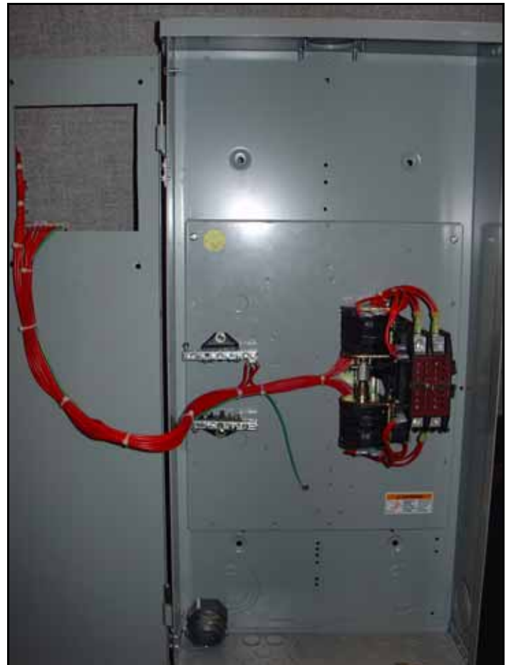
Figure 6. Typical Power Panel for 100 A Model.
