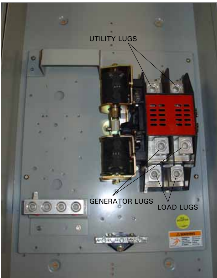
Figure 13. Cable Connection Locations (200 A).
