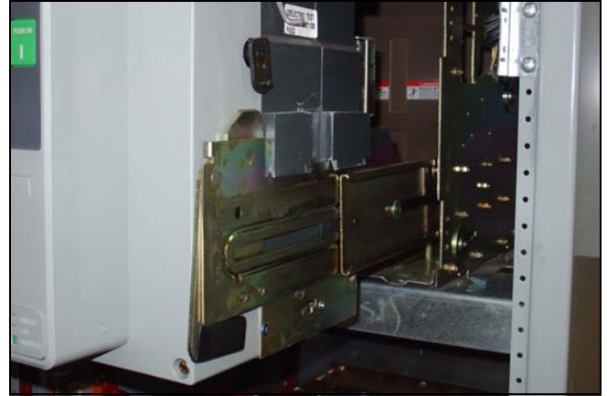
Figure 28. Switching Device in the REMOVE Position.
