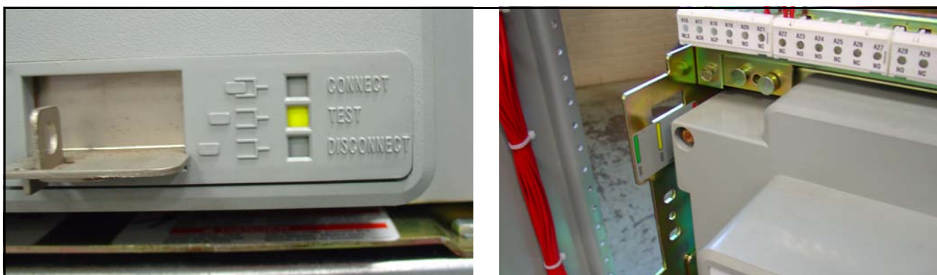
Figure 30. Switching Device in the TEST Position.
