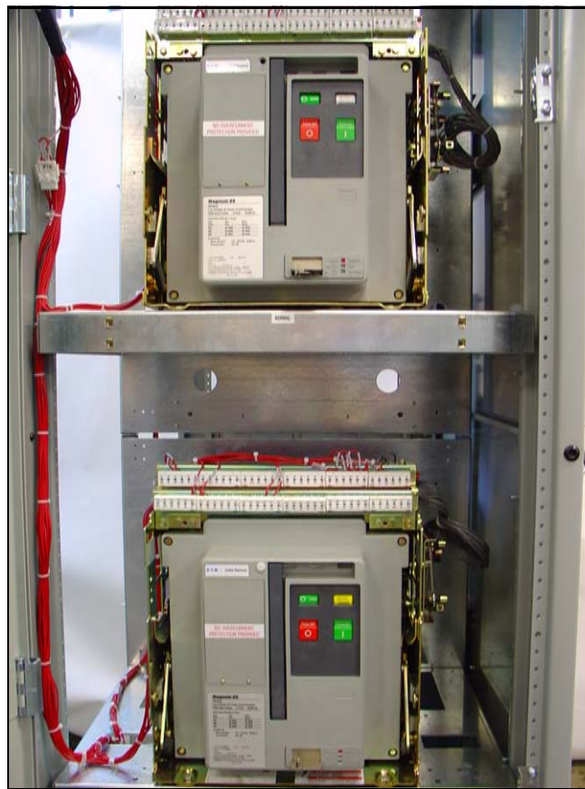
Figure 11. Typical Power Panel (Open Transition Shown).
