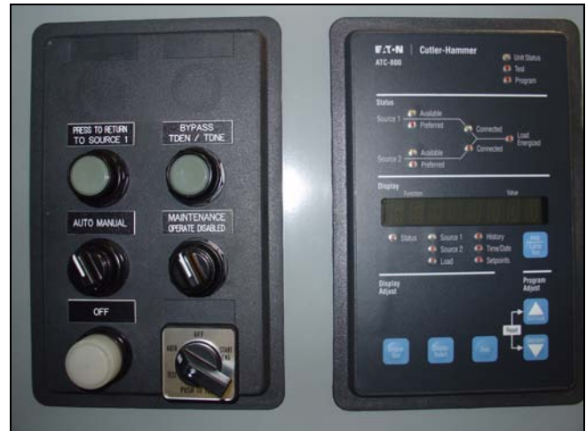
Figure 35. Bypass Isolation Switch.
