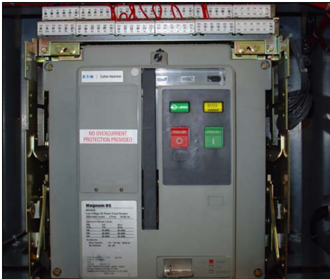
Figure 8. Drawout Switching Device Installed in the Magnum Transfer Switch.
