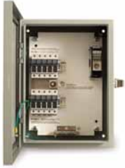
DC combiner boxes
