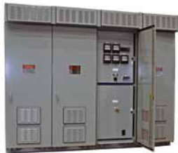
Medium voltage AC switchgear
