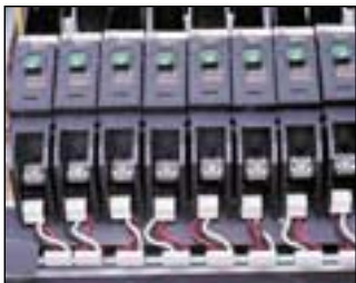
Cutler-Hammer Smart Breaker™ technology provides reliable and flexible lighting control.
